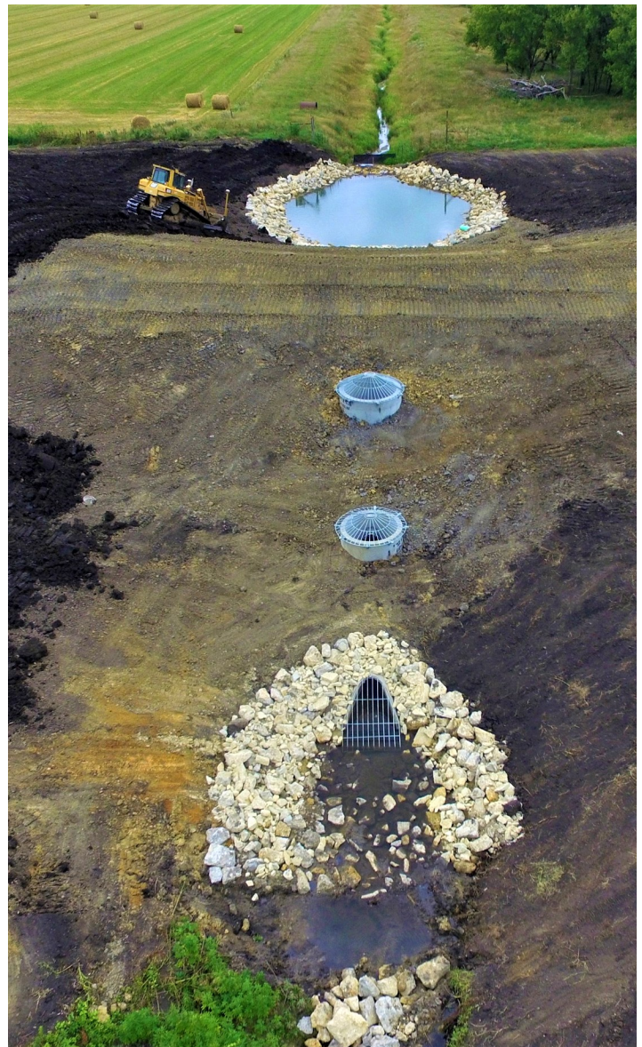
Work progresses Aug. 3, 2020, at the Dexter 30-Dam 2 project site in the headwaters of the South Branch of Dobbins Creek.
