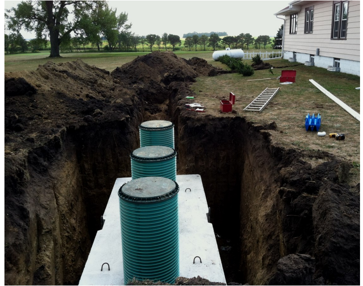
An area contractor installs a new subsurface sewage treatment system (SSTS) during the summer of 2020 in the Cedar River watershed.
