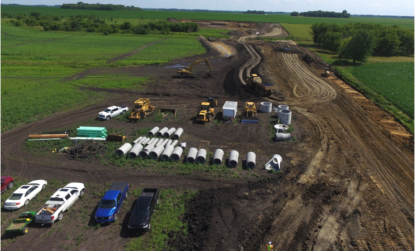
Crews work July 1, 2020, to build CRWD's biggest, CIP upland-storage berm to date in the headwaters of Dobbins Creek's south branch.
