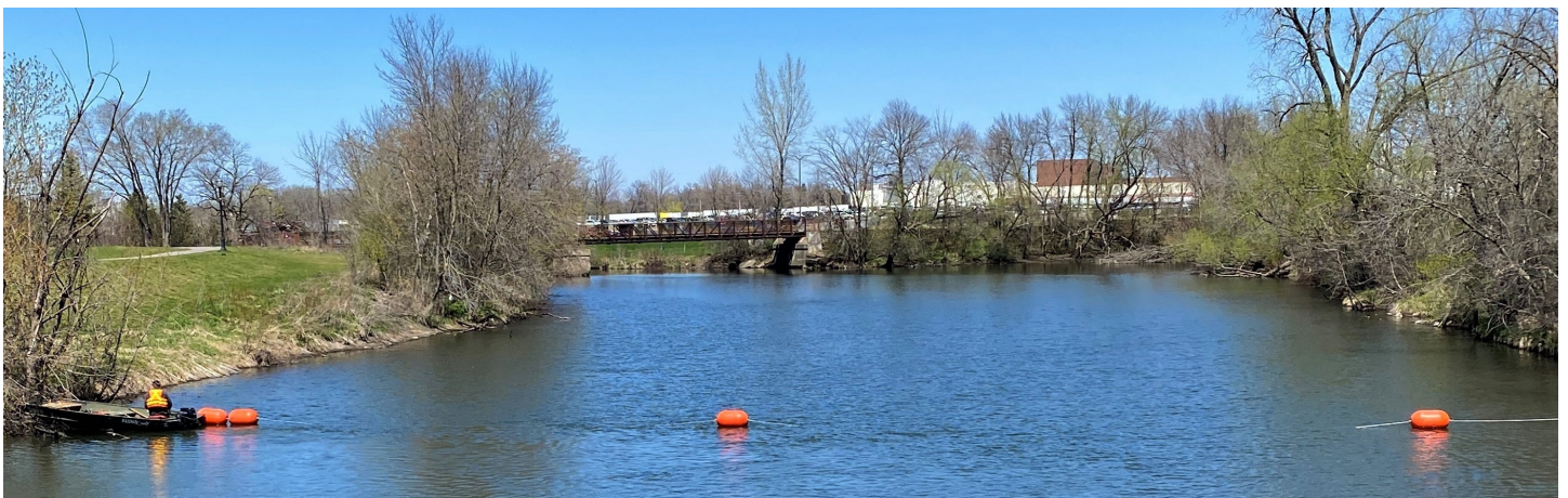
MN Dept. of Natural Resources installs a barrier float in April 2020 on the Cedar River State Water Trail to enhance boater safety above Austin's downtown dam.
